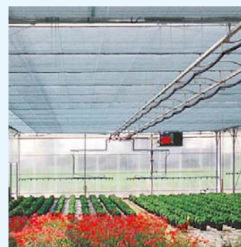
Irrigation boom in a greenhouse with thermic screen . Upper-bar omega shaped due to the heating system.
